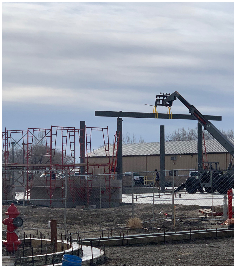
CC Communications new location under construction on S. Maine Street due to finish construction on December 2021.
