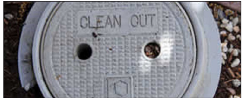
Cleanout vent that should be sandbagged if in a flood-prone area. Photo by Rachel Dahl.
