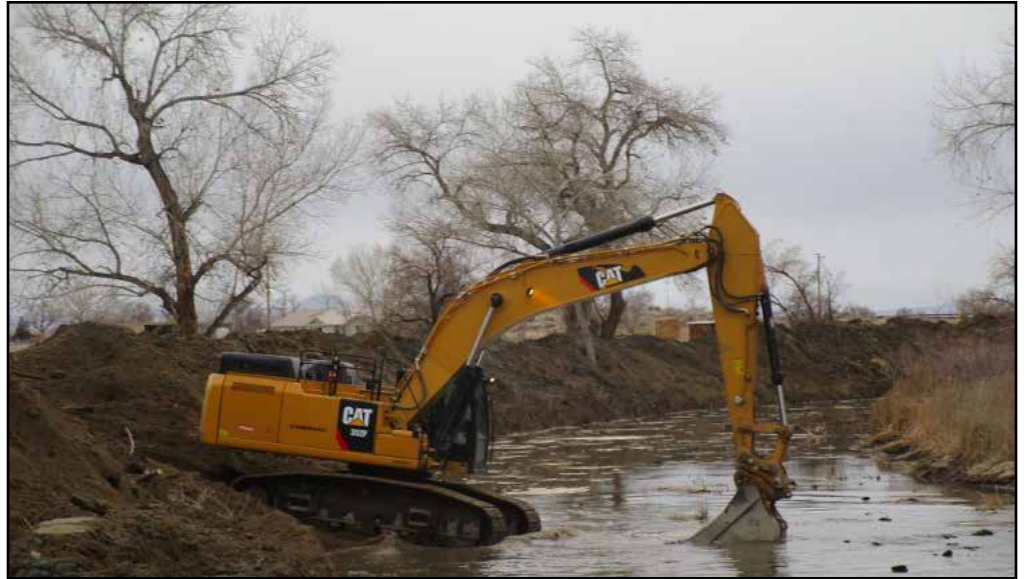
Cleaning debris out of the Carson River in 2017. Similar actions begin the week of March 6 as the county prepares for potential heavy snowmelt.
